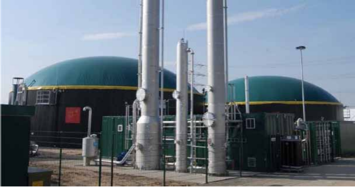
Biogas feed-in system to the natural gas grid: pressurized water cleaning and transfer station
