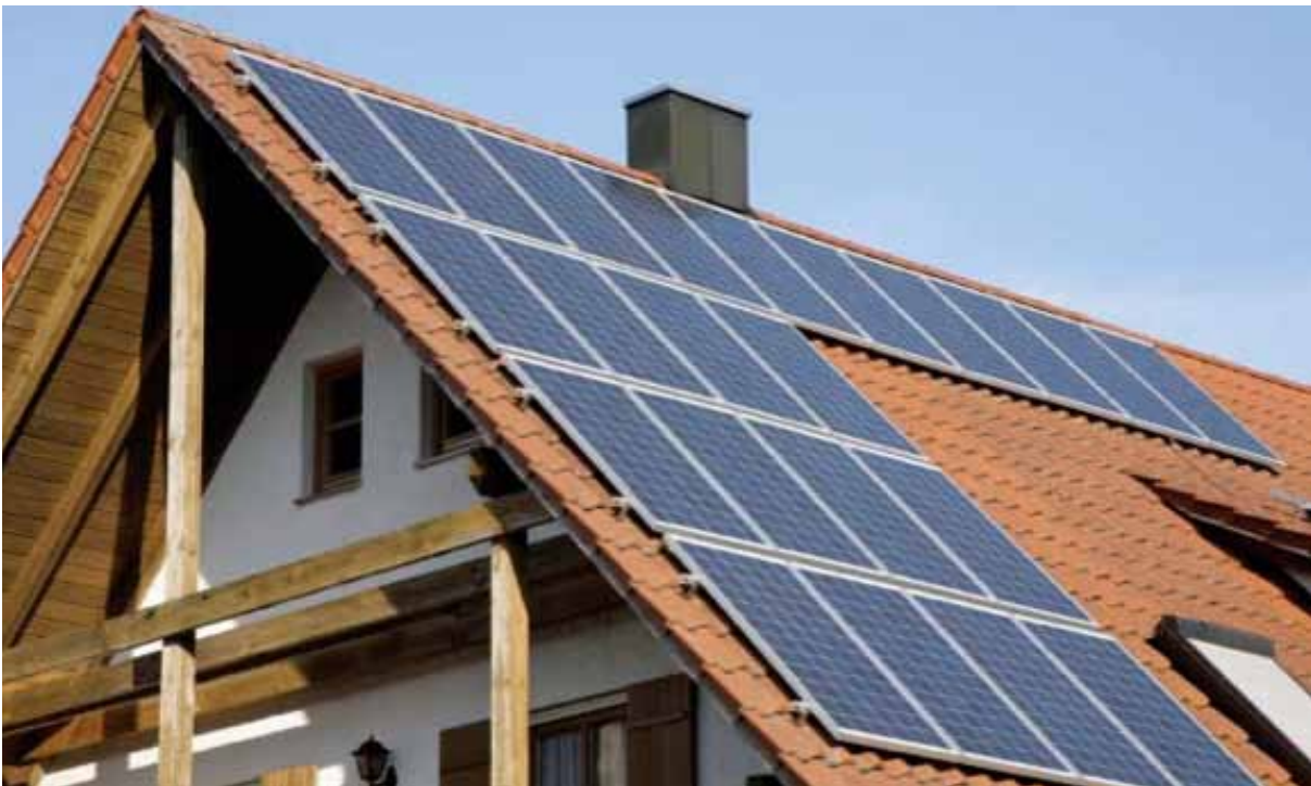
Photovoltaic roof systems
